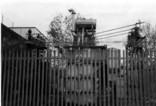
33/11 kV TRANSFORMERS AT BRIDGE STREET
