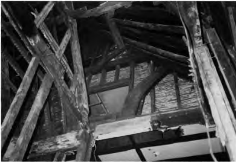
GABLE END OF ROOF OF FORMER BLACKSMITH'S SHOP, GREAT BOOKHAM, LOOKING FROM THE SOUTH-EAST.
