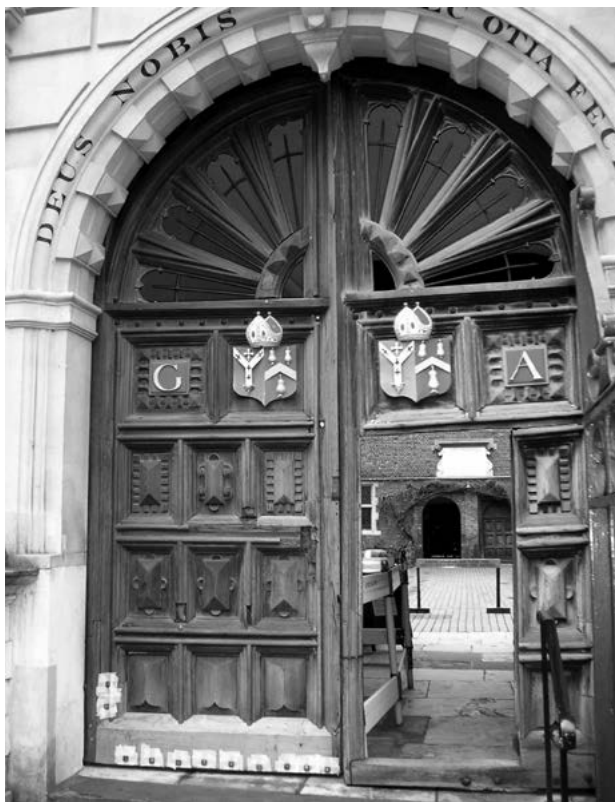
Abbots Hospital, Guildford – Repairs funded in part with a Surrey Historic Buildings Trust grant
